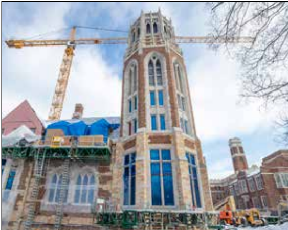
Crews are nearing the completion of the E. Bronson Ingram College, Vanderbilt's newest residential hall for on-campus student housing.
